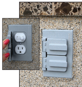
Light Switch & Extra Electrical Outlet
